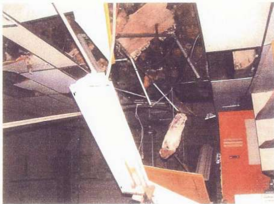
Ceiling Degradation in Bldg 2000 Room 29
