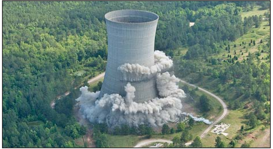
The massive structure is the second largest cooling tower to be demolished worldwide.
