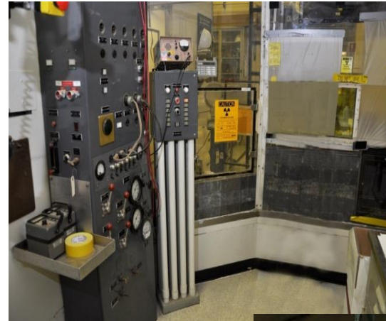
RC-1 Hot Cell Sample Access Port
