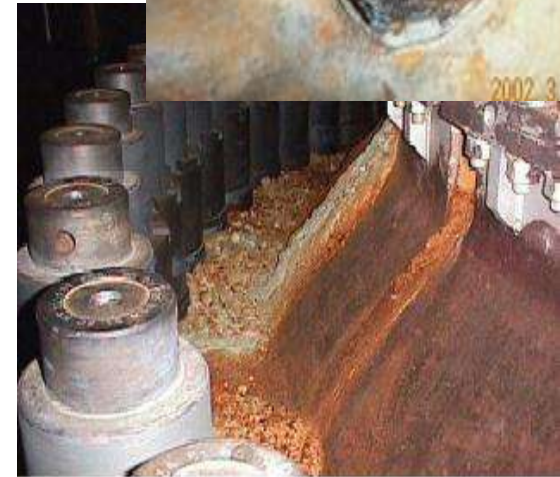
Red Rusty Boric Acid Deposits on Vessel Flange (12RFO)
